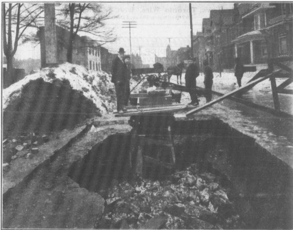
BREAK IN SEWER, ROBERT STREET, TORONTO.
