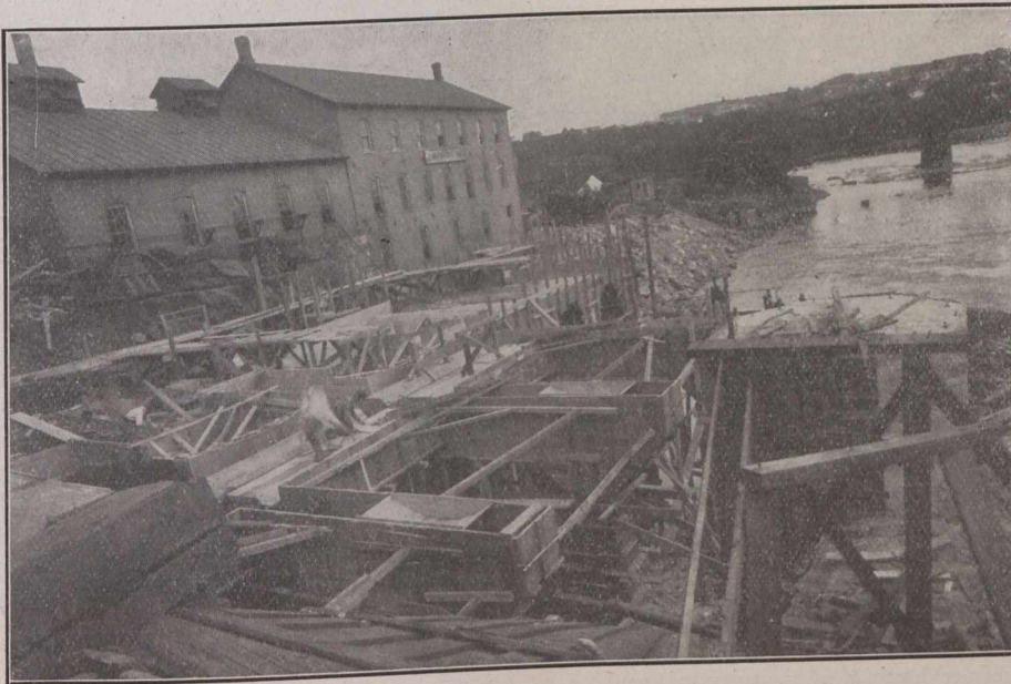
Site on Magog River, showing Foundation Work of New Power Development Being Erected By Sherbrooke Railway and Power Company.
