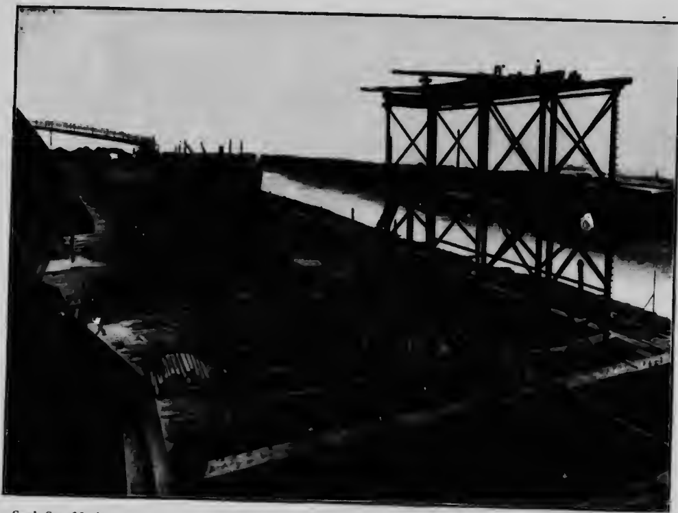
Sault Ste. Marie, Ont.—Lake Superior Corporation—Cold storage yard, dock and coal-unloader. 650,000 tons of coal will be handled over this dock annually during navigation.
