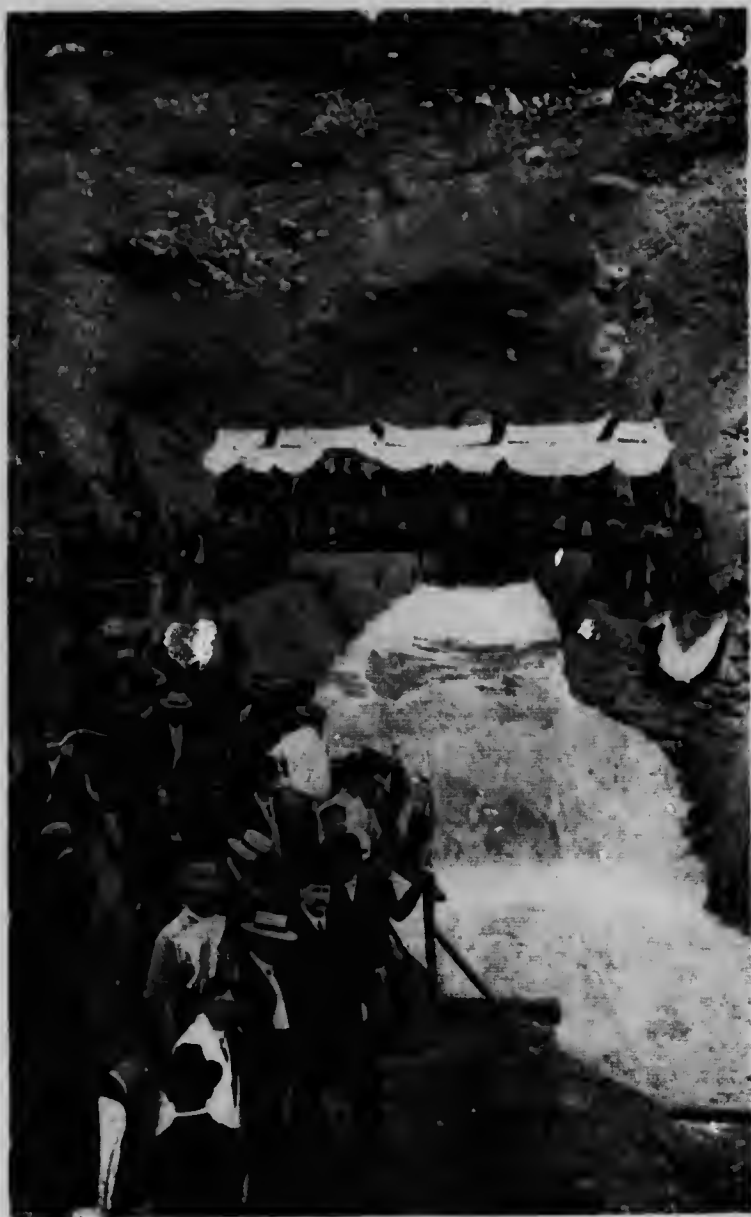
Commission of Conservation.—Vancouver Power Company—Opening of tunnel connecting Coquitlam's and Bucatzen Lakes.
