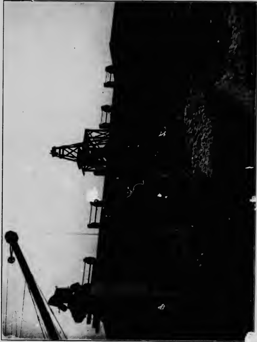
The Intake, Southern Alberta Land Co., Ltd., Canal—Five steel gates each 8 feet high by 10 feet wide.
