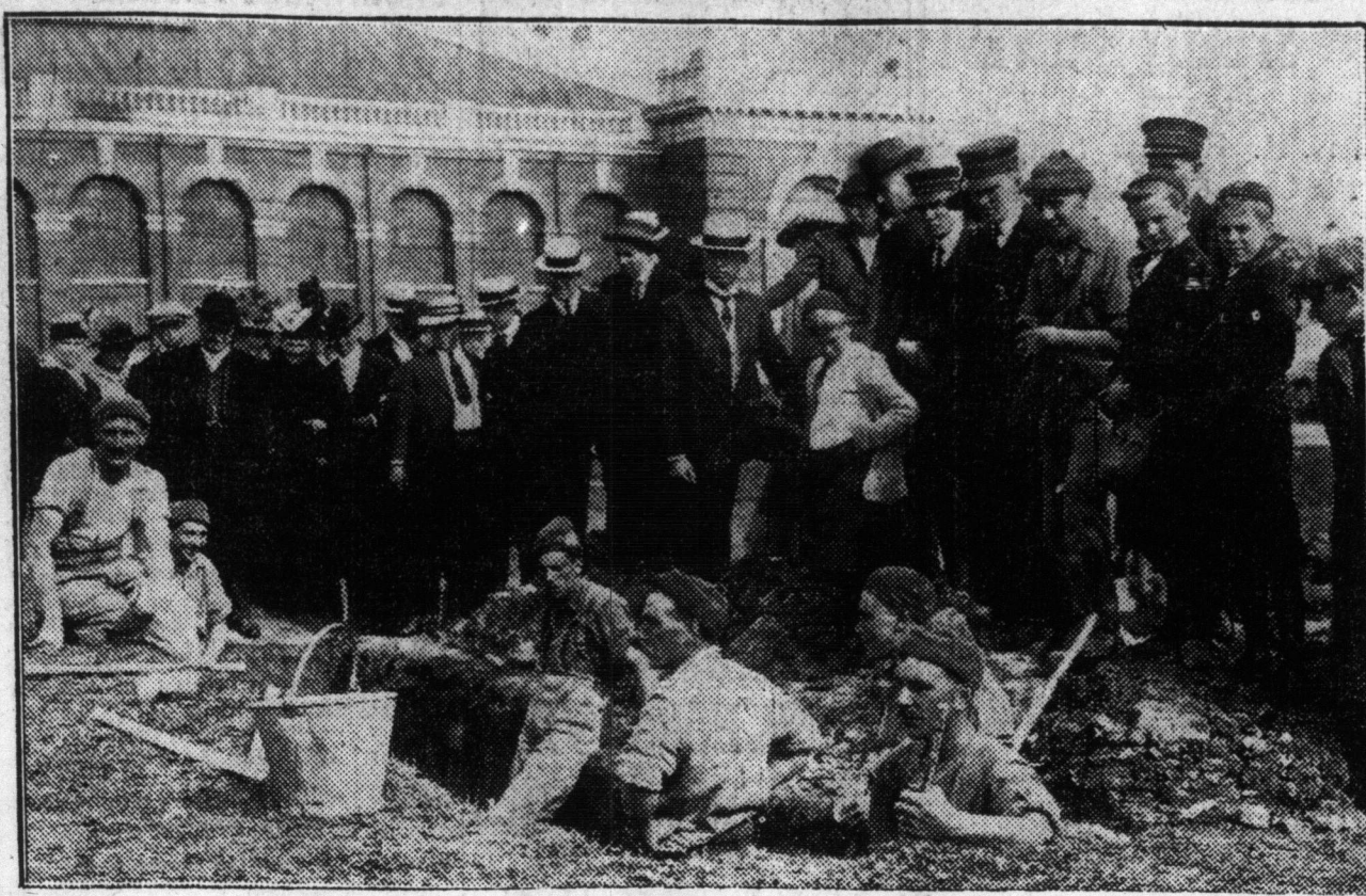
Exhibition of trench digging given by members of the Canadian expeditionary force now camping on the Exhibition grounds.
