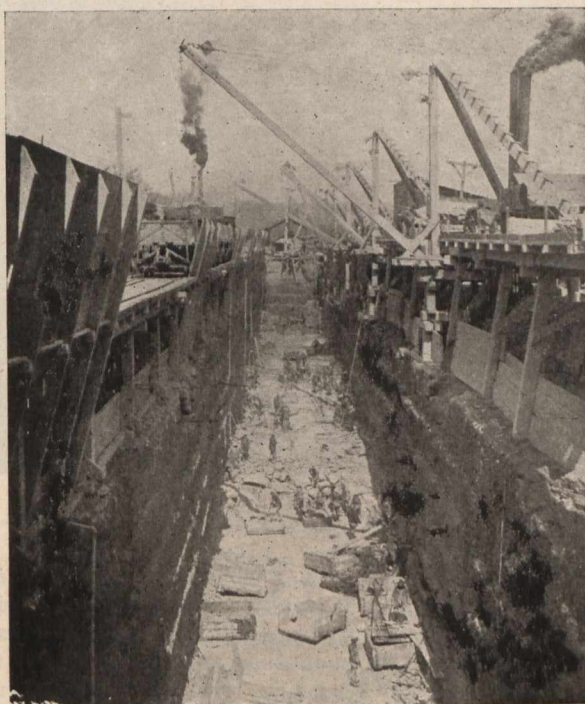
Toronto and Niagara Power Co. From a photo taken May, 1904, showing progress of excavation work in wheel pit.
