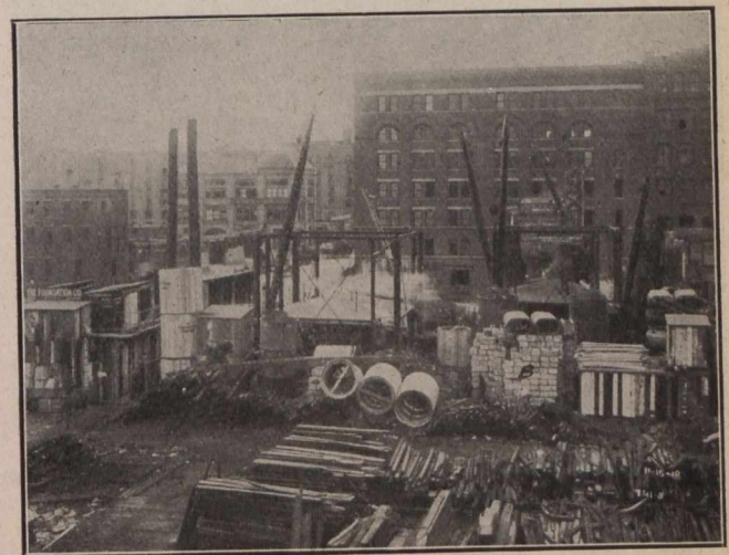
Fig. 2.—Showing Two Four-Masted Steel Derricks. Steel Forms used for Building up Cylinders—Collapsible Steel Shafts Inside of Steel Forms. Wooden Cofferdams, Used where Concrete Stopped Below Ground. Pile of Cast Iron Blocks Marked "B" Used for Weighting Down Caissons. Each Block Weighs 1½ to 2¼ Tons.
