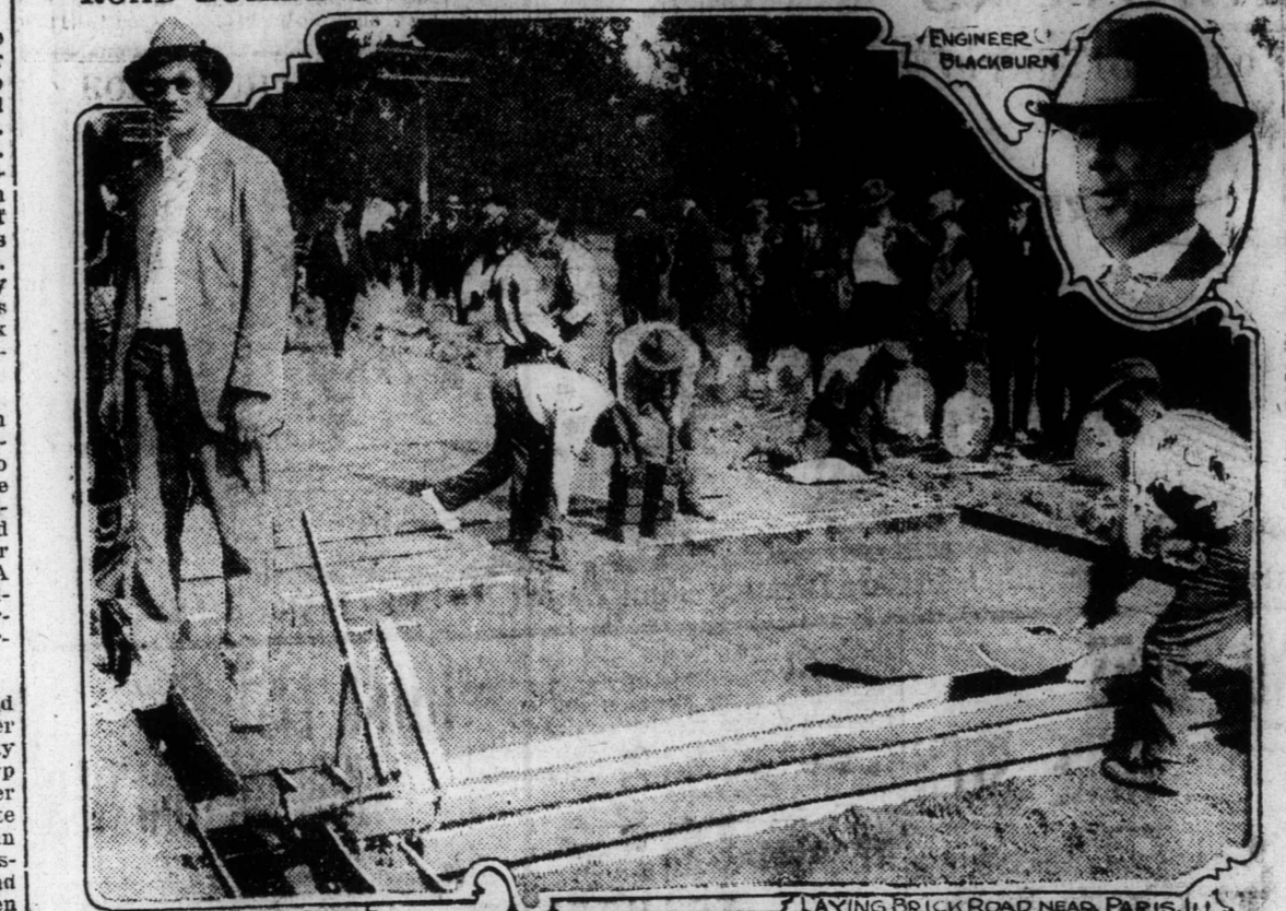
For the first time in the history of road building in America, theory of construction was transferred from the inside meeting place of engineers to the field of practice upon the highway by 300 engineers and contractors when they came together recently at Paris, Ill., to witness the manner and method by which a monolithic brick road is built. The method of laying brick in the green concrete was demonstrated in detail by the execution of every step from the preparation of the roadbed to the completion of the pavement. The machinery used and method of performing the work upon the construction was credited to Engineer W. T. Blackburn and Contractor Alan Parrish, under whose supervision the exhibit was displayed. Among the spectators were members of highway departments of seven states, while representatives from universities numbered more than two score. Editors of engineering journals especially displayed great eagerness in observing details of construction about which they have written in the past so approvingly. Others present were those deeply interested in the economic problem of road building that is now so acute with every user of the highways. All of these visitors expressed a deep appreciation for this unusual opportunity and particularly for the economical methods strongly apparent. The convictions which will be carried back to various sections concerning economy in road building as expressed by many of those present will save to the country 7 thousands of dollars, as a thing seen is believed to be without doubt or foreboding.
