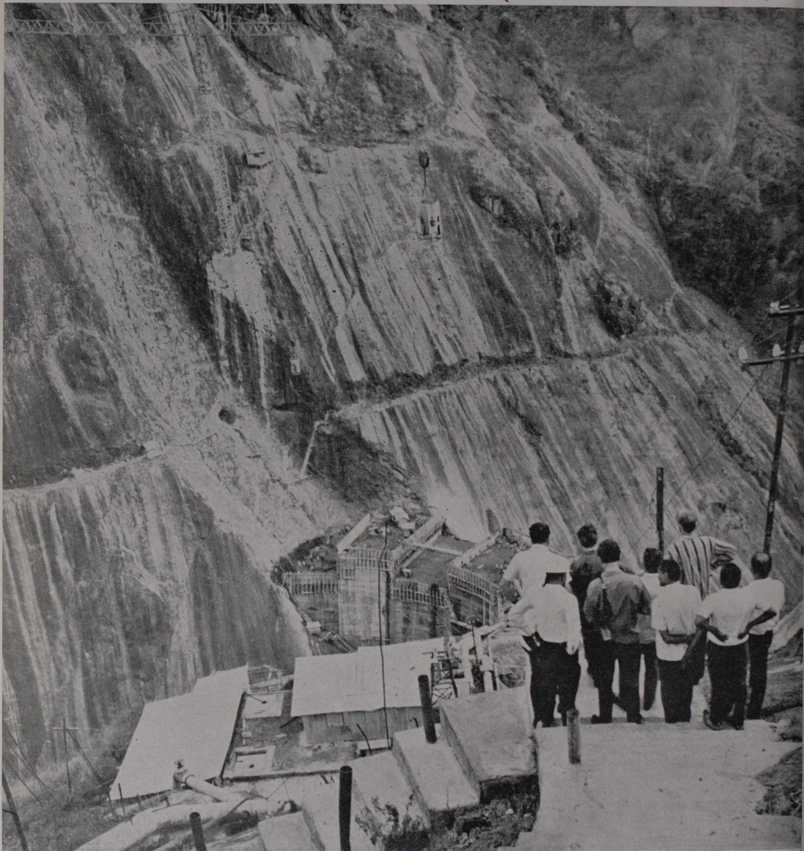
Mr. Gerin-Lajoie viewing the Idikki Arch Dam. Located on the western side of the Nilgiris, in Kerala, the project is changing the face of the Periyar Valley. With an installed capacity of 780MV (for peaking), Idikki will be the biggest hydro-electric scheme in South India. The 560 feet high arch dam will be the first arch dam in India and the highest in Asia, over three times the height of Niagara Falls. Besides cheap power, the project will irrigate 150,000 acres via canals downstream.
