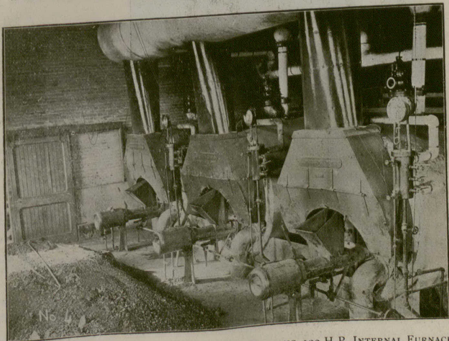
FIG. 6.—VIEW OF PORTION OF BOILER ROOM, SHOWING 100 H.P. INTERNAL FURNACE BOILERS WITH UNDERFEED STOKERS AND PORTION OF STEAM PIPING.
