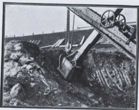
A STEAM SHOVEL WILL LOAD A TRAIN OF FLAT CARS IN A FEW MINUTES
