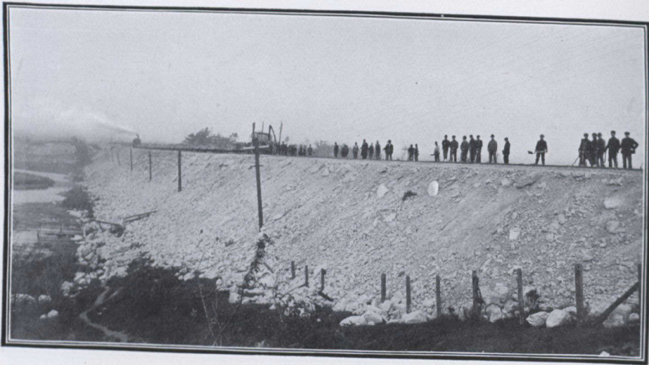
"RIVER ROUGE FILL" ON GRAND TRUNK SYSTEM, 17 MILES EAST OF TORONTO. THE HARD PAN OUT OF HOG'S BACK CUT WAS USED TO RAISE THIS BIT OF TRACK TWENTY FEET. IT IS RAISED STEADILY FOOT BY FOOT, CONSTRUCTION AND OTHER TRAINS PASSING OVER IT ALMOST AS USUAL.
