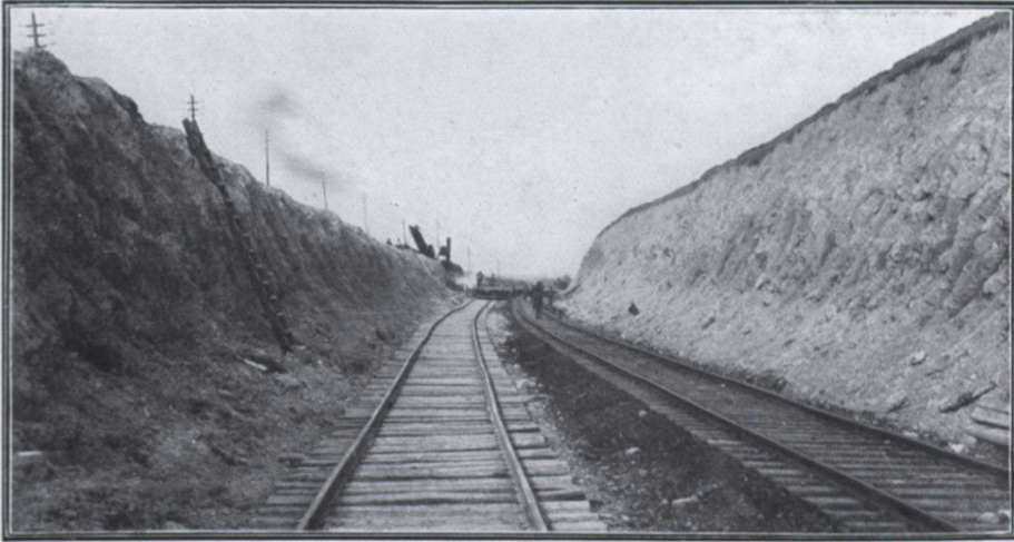
ANOTHER VIEW OF THE "HOG'S BACK" CUT ON GRAND TRUNK, SHOWING THE CUTTING AS IT APPEARED AFTER BEING LOWERED 22 FEET, AND PREVIOUS TO THE FINAL CUT OF THE SHOVEL. THE CUT IS WIDE ON ACCOUNT OF THE DOUBLE TRACK
