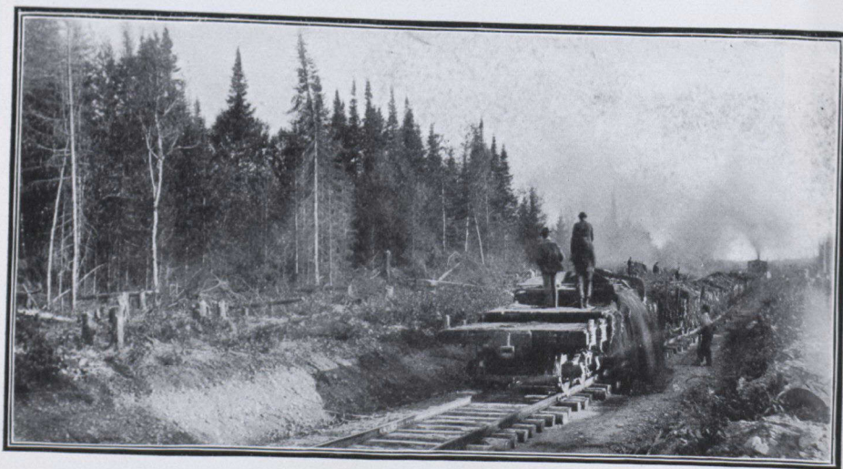
BALLASTING A BIT OF NEWLY-LAID TRACK. AN UNLOADING PLOUGH IS CARRIED ON THE REAR CAR. A CABLE CONNECTS IT WITH ENGINE. BY IT A TRAIN IS UNLOADED IN A FEW SECONDS. THE T. AND N. O. RAILWAY.—PHOTO BY PARK, BRANTFORD
