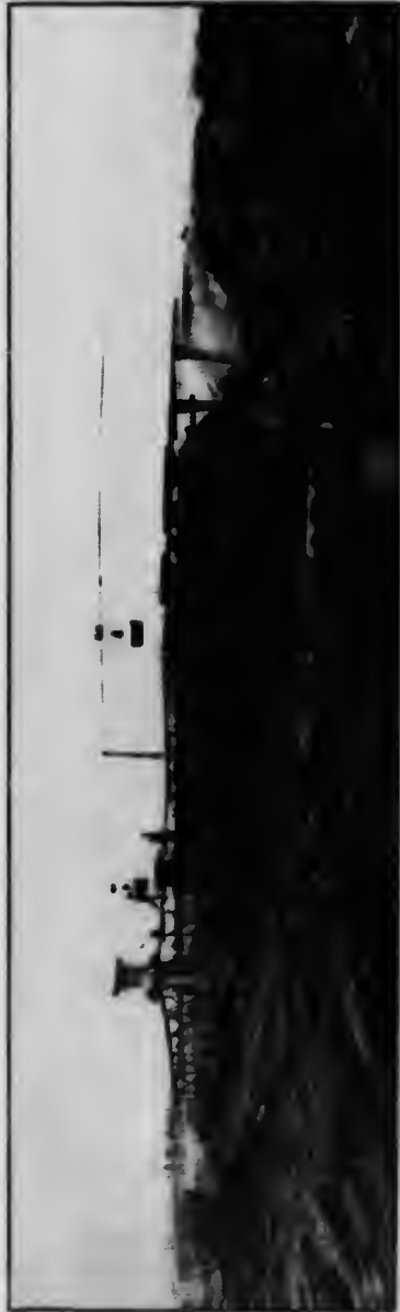
ROAST YARD AT VICTORIA MINES, MONSIEUR NICKEL CO., SHOWING METHOD OF CONSTRUCTION OF ROAST HEAPS.
