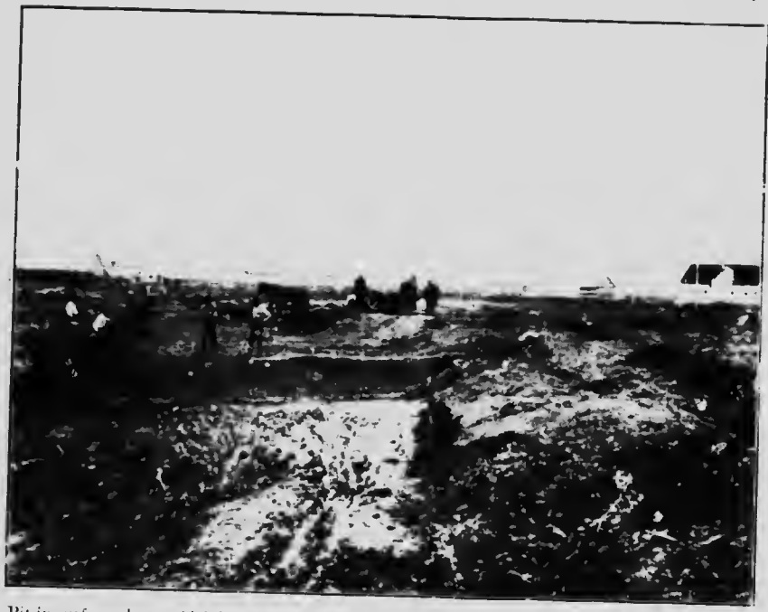
Pit in surface clay at Alsip's brick plant, Winnipeg, Man. The pit has been excavated in the calcareous surface clay and the bottom of the excavation represents the top of the underclay.
