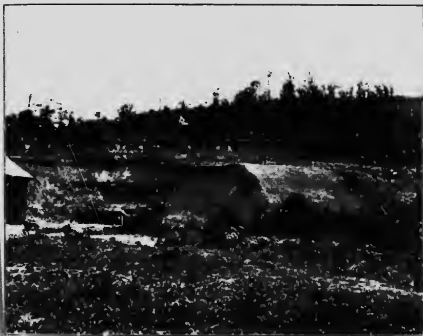
Bank of decomposed Nidnara shale, used for dry press bricks. Leary, Min.
