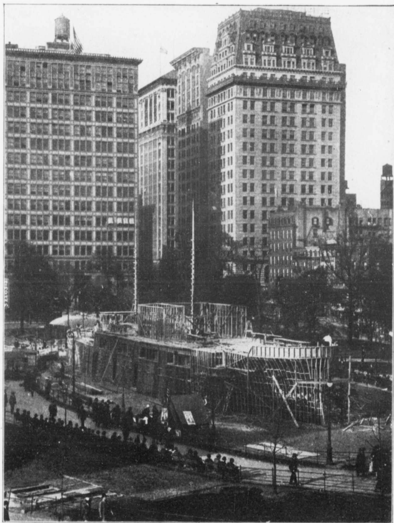
A 250-foot battleship being erected in Union Square, New York City, for a recruiting station.
