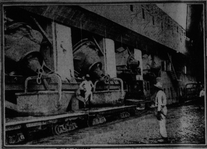
This photograph was taken in the great concrete mixing works on the hilltops overlooking the Gatun dam—it shows one of the batteries of mixers.
