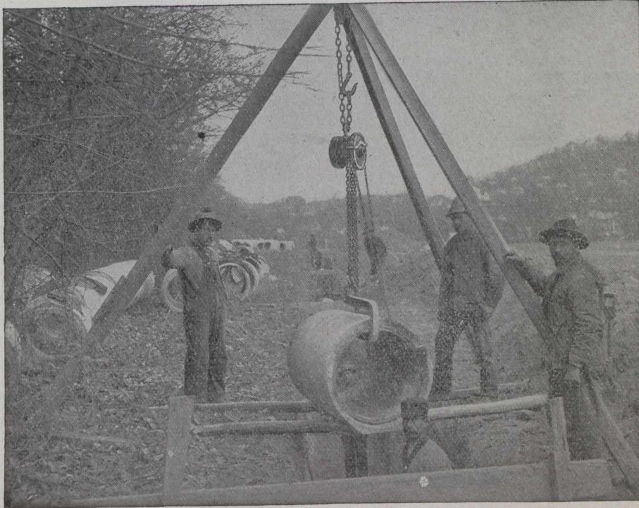
A Triplex Block hung from a temporary rigging and used for laying pipe.
