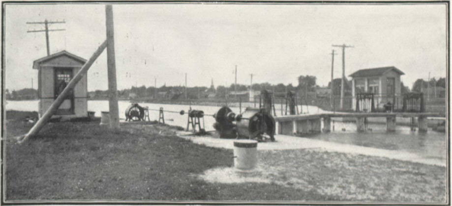
CORNWALL—SHOWING THE MACHINERY OPERATED BY ELECTRICITY, USED TO OPEN AND SHUT THE GATES AND THE SLUICES
