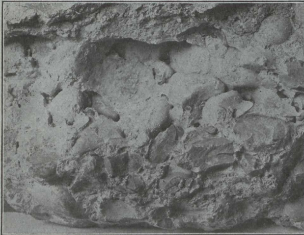
Fig. 2.—Block Cut from Pavement, Showing Segregation of Stone and Bridging Effect
