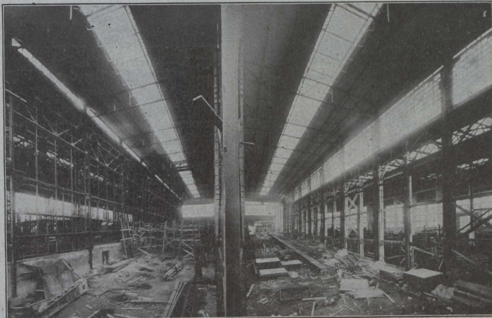
Fig. 1.—Interior View of Berth, Showing Both Sections. Looking Toward Land End. Beyond Columns at the Left is Another Covered Steel Berth. Beyond Columns at the Right is a Covered Wooden Berth
