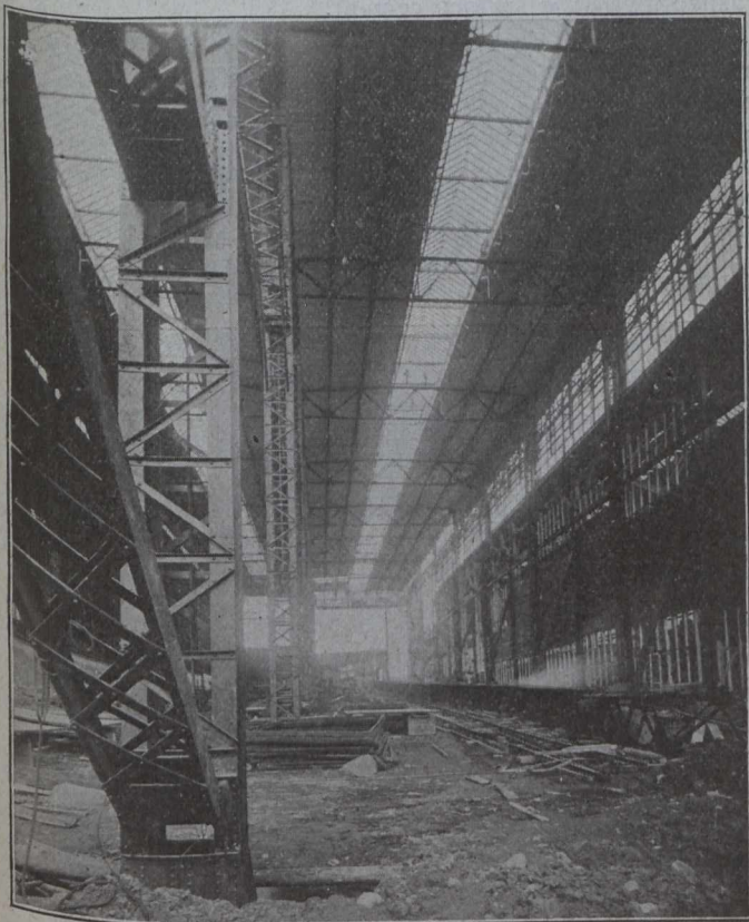
Fig. 5.—One Section of Completed Berth, Looking Toward Land End. Note Preparation for Laying Keel of Ship
