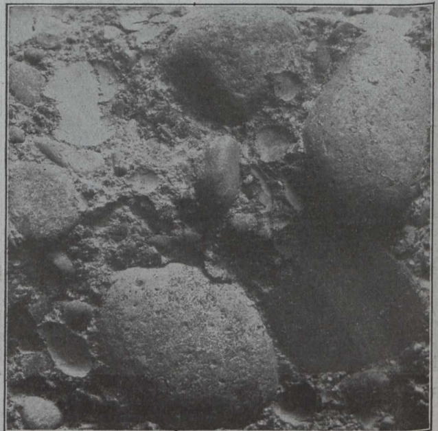
Fig. 3.—Fractured Surface of 6-in. Cube, Showing Effect of Segregating Coarse Aggregate
