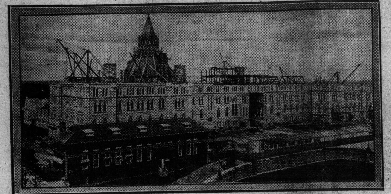
Photograph showing progress made on the reconstruction of the parliament buildings at Ottawa. Work was started one year ago, and as no work was done during the winter this represents eight months' building.
