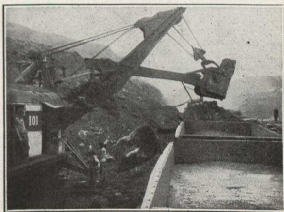
Steam Shovel at Work in Culebra Cut, with Large Rock in Mouth of Shovel.
