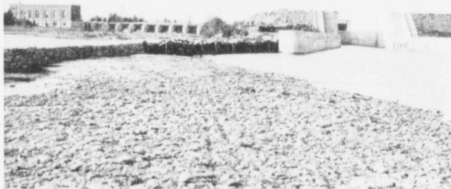
ONTARIO HYDRO-ELECTRIC POWER COMMISSION - HYDRO-ELECTRIC PLANT, FRANKFORD, HASTINGS CO., ONT., CENTRAL ONTARIO SYSTEM, TRENT CANAL.
