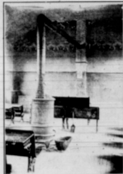
The school room as it was. Note the broken plastering, hanging wall paper, projecting floor and ill-arranged furniture.
