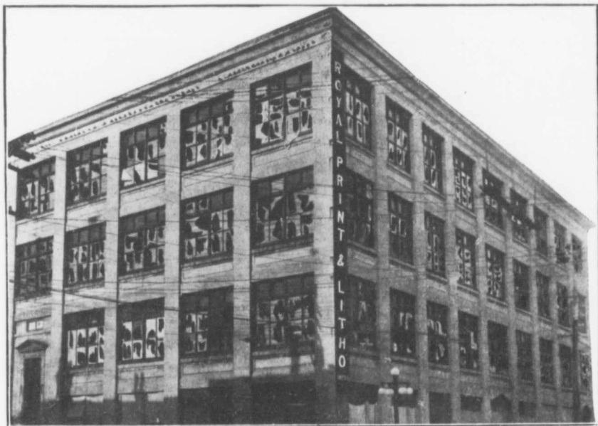
THE HOME OF THE ROYAL PRINT & LITHO LIMITED AFTER THE EXPLOSION. This building is situated more than two miles from the scene of the disaster, and so great was the explosion that every window was shattered. Temporary repairs were completed and business resumed with but little delay.
