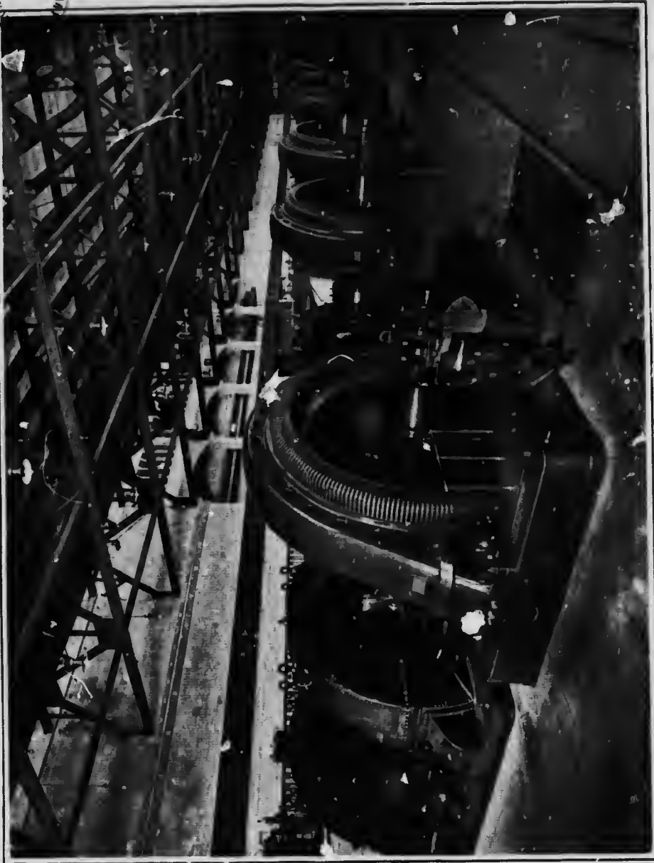
Interior of the Generating Station, Ontario Power Company.
