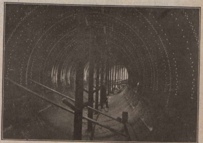
FIG. 2—DOUBLE-RIVETED LAP JOINT IN 18-FT. DIAMETER PIPE, ONTARIO POWER CO.
