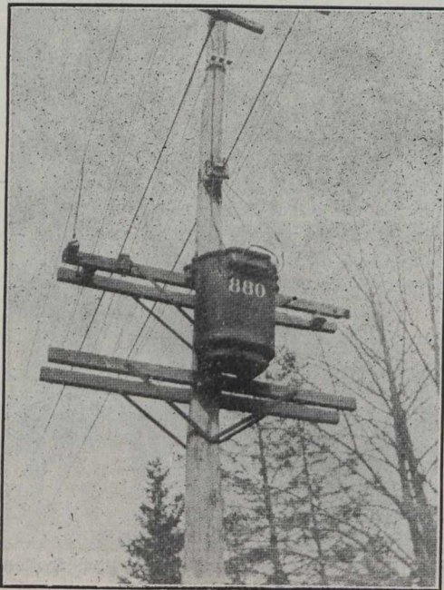
Fig. 6.—Single Primary Fuse Block.
