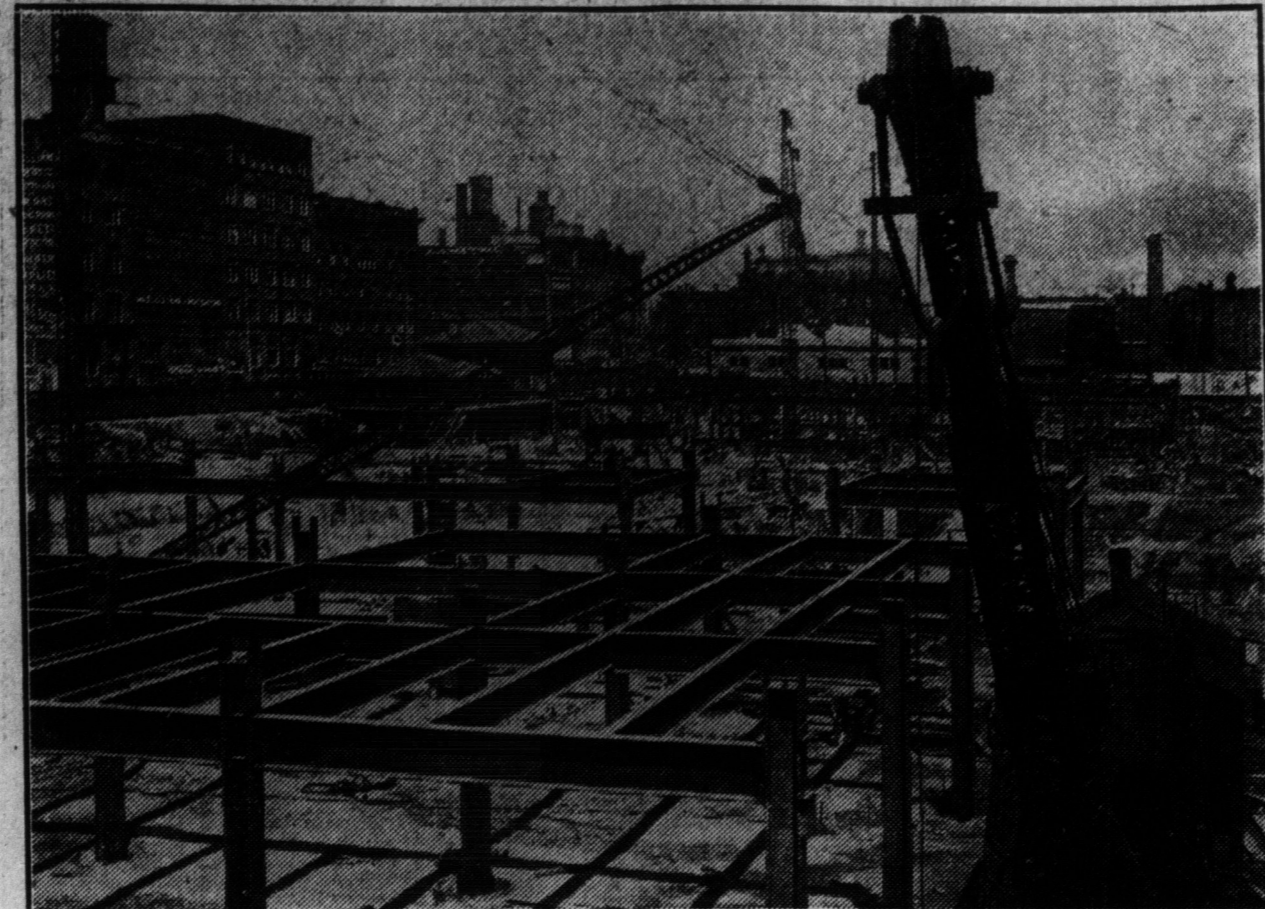
The new Union Passenger Station on Front street from York to Bay streets. Cut shows first storey of steel pillars that will carry the structure. The Custom House is in the upper field, right of the center line.
