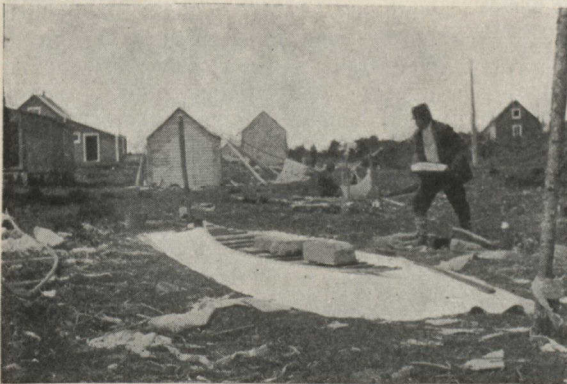
THE TEMPORARY FRAME BEING WEIGHTED DOWN ON TOP OF THE CANVAS WITH ROCKS
