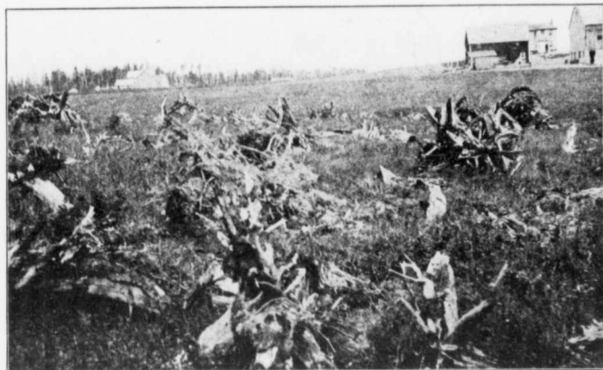
All stumps removed and made ready for piling. Horsepower and powder were the means used to remove these stumps.
