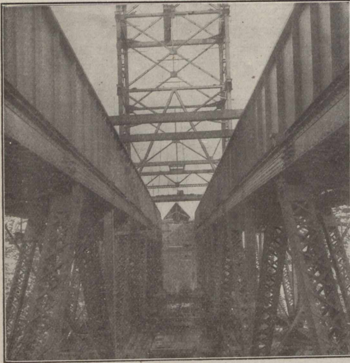
Fig. 6.—North approach span erected. As the railway tracks on the bridge are 32 ft. centre to centre, these approach spans are erected as two separate bridges, each carrying a track.
