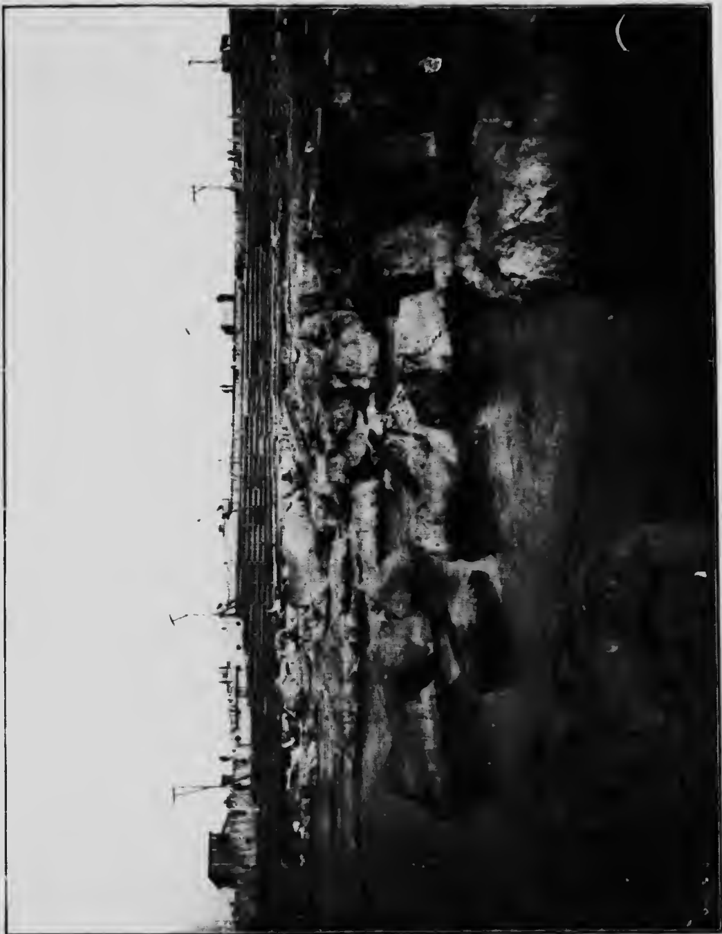
Photograph showing successful unwatering of Cascade rapids between the main and subsidiary Coffey Dams. On the farther side of the main Coffey Dam is the most turbulent rapid in the Upper Niagara River. The contour of the river bed gives some idea of the difficulties experienced in securing stable foundations for the Dam. The depth of water encountered at this point was fourteen to fifteen feet.
