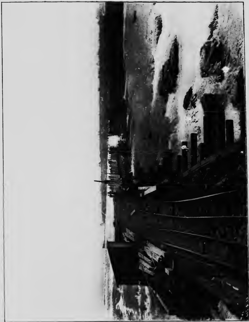
Photograph of Main Collier Dam showing arched form of construction. A double track line of standard gauge is used to bring materials required in construction, such as timber, rock, clay, etc.
