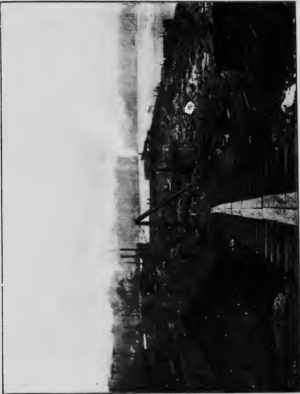
Site of Power House and Wheel Pit, surrounded by subsidiary Coffler Dam. The Wheel Pit Excavation will be covered by a rough building so that construction can proceed night and day irrespective of the weather. This site was covered by water to an average depth of 7 feet.
