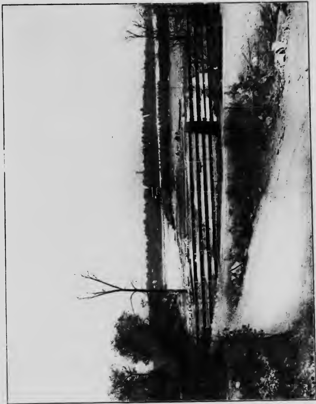
Photograph showing arch construction of main Cedar Dam, which adds materially to its stability. From the end anchored to the shore to the end under construction at the foot of second cascade it will be seen that the arch form of construction has been maintained.
