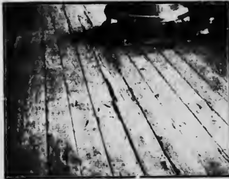
FIGURE 62.—Floor full of cracks.
