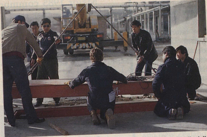
Technicians from Canadian Scale Company Limited in Toronto install a fully electronic in-motion truck scale system in a coal handling facility in Taiyuan, Shanxi, People's Republic of China. It is the first of its type to be installed in the country.
