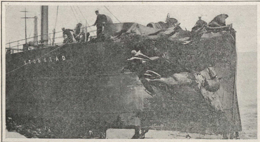
When the Storstad's bow, with the grim impact of 11,000 tons of coal at full steam ahead did her work, she apparently got a wrench to starboard.
