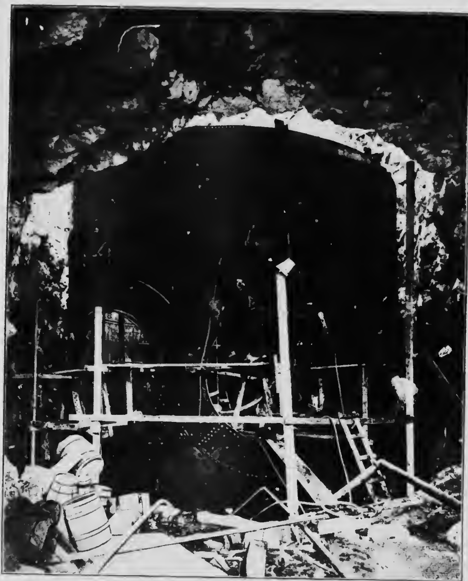
Plant No. 2, Lake Buntzen. View of Surge Tank showing openings for pipe line connection
