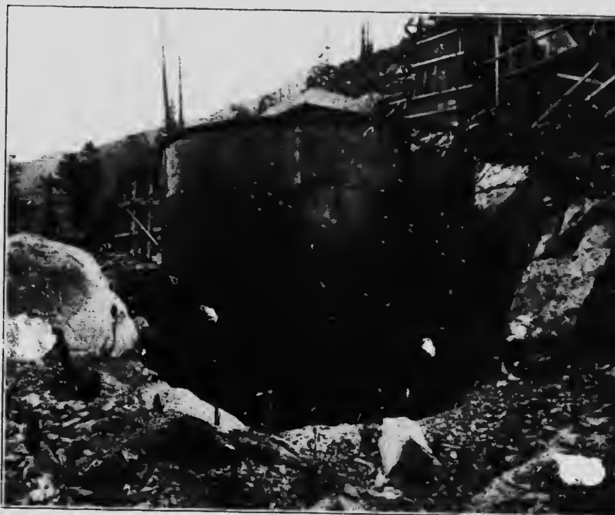
Plant No. 2, Lake Buntzen.—Top of Surge Tank.
