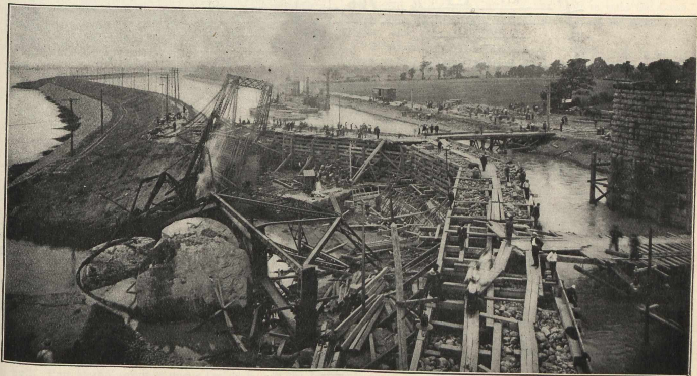
View of Repairs to Cornwall Canal.—View Looking West, July 4th, Eleven Days After Break.
