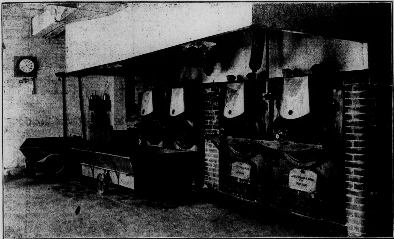
Battery of Roasters (incomplete) in Chase & Sanborn's New Factory. Two more Roasters to be installed.
