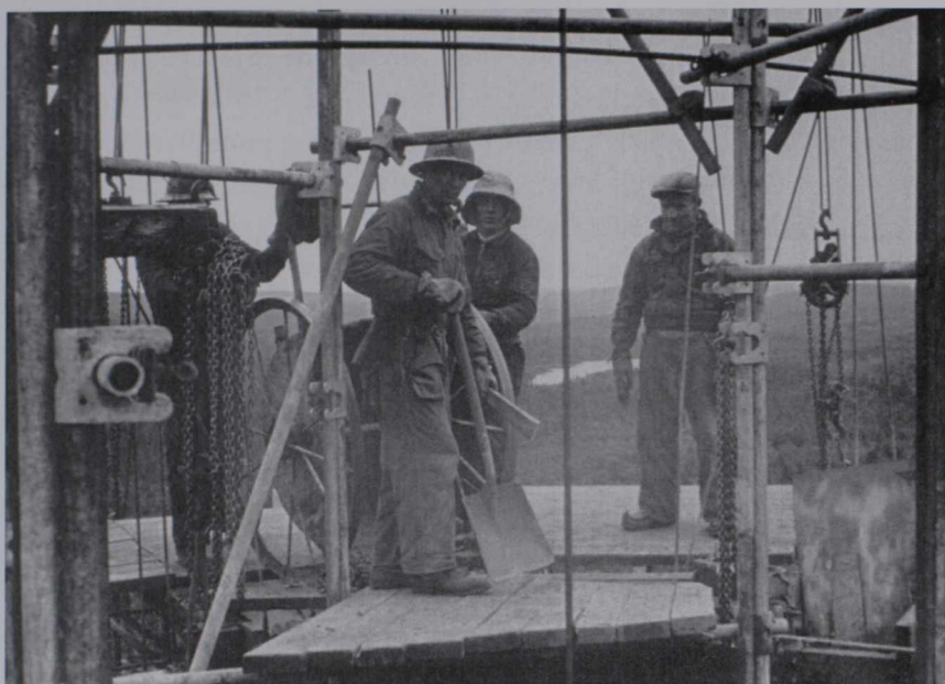
Kolosjoki nickel and copper mine. Workers on scaffolding. Photo: Kalervo Rankama, 1939. Source: Open licence of the Geological Survey of Finland.
