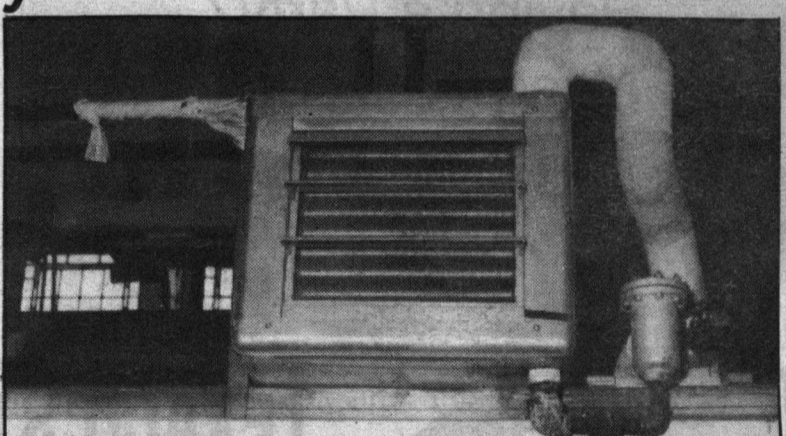
One of the heaters in Art Workshop 3 suspected of blowing asbestos into the airstream.
