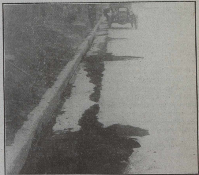
Failure at Curb.
