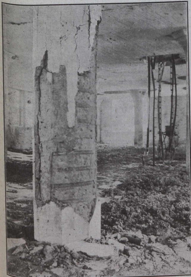
Fig. 14—A Few Light Blows with a Hammer will do this to an Apparently Whole Column owing to Dehydration of the Cement by the Extreme Temperature of this Fire.
