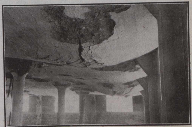
Fig. 11—Sagging Floor Slabs are at Point of Incipient Failure.
