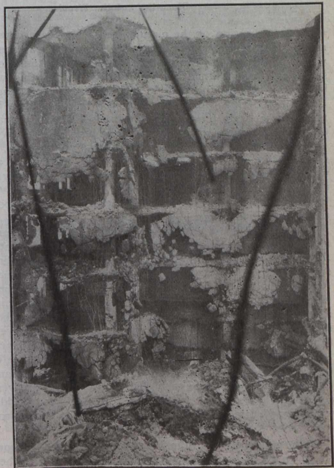
Fig. 6—Looking Directly Toward Standing 1\frac{1}{2} Bays to the north. View taken from Standing Bays at the south end.
