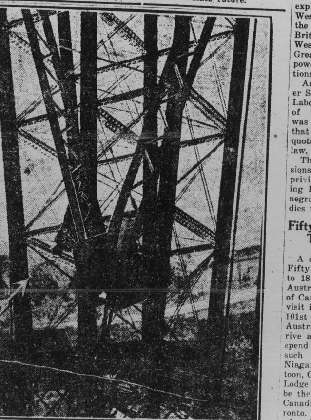
An iron worker photographed a hundred feet above the Niagara River while working on the Canadian end of the Michigan Central bridge now in the course of erection.
