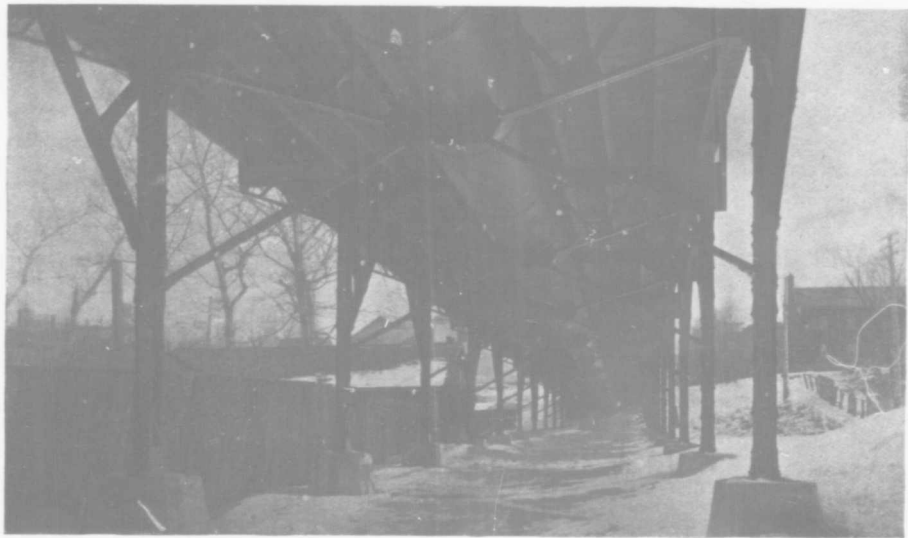
LONDON SEWERAGE SYSTEM. KING STREET VIADUCT. SHOWING CONSTRUCTION OF STEEL PIPE AND FLOOR-BEAMS.
