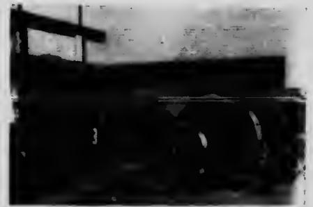
INTERIOR VICTORIA AVENUE TRANSFORMING STATION.
