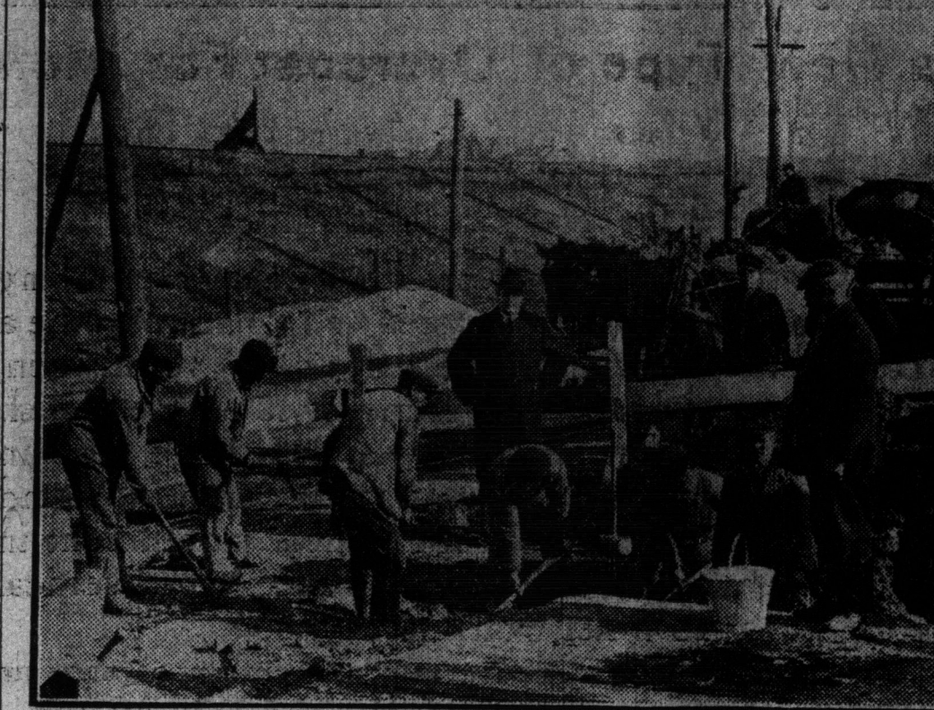
Work commenced yesterday on the filling in of Catfish Pond, and by next spring residents of the High Park district will not know the place.
