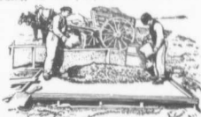
The mixing and placing of concrete is simple, and is easily learned. No elaborate tools are needed.
