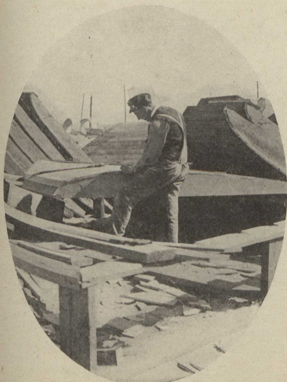
Making the Wooden Moulds that shape the Cement Floor for the Filtration Beds.
