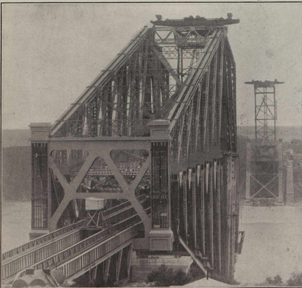
General View of Present Stage of Erection of the Quebec Bridge (taken from the North Shore).
