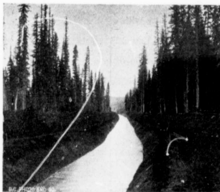
Cut, 10 feet deep and ¼ mile long, excavated to open Polleys Lake.
