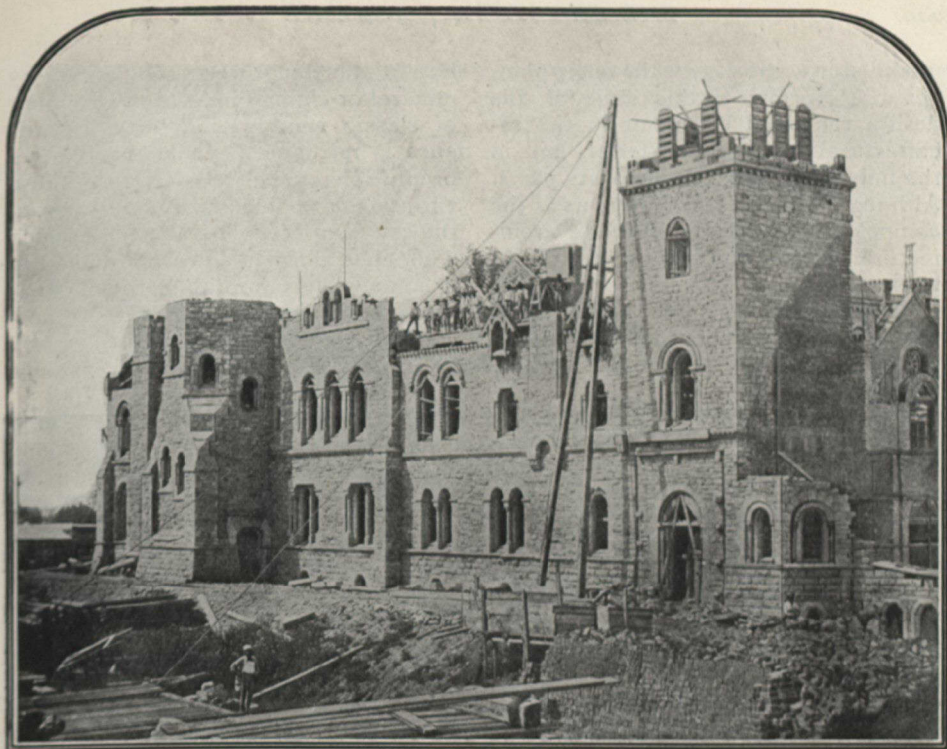
VIEW OF THE BUILDING OPERATIONS, TAKEN FROM THE NORTH-EAST, SHOWING THE TWO EASTERN ENTRANCES
