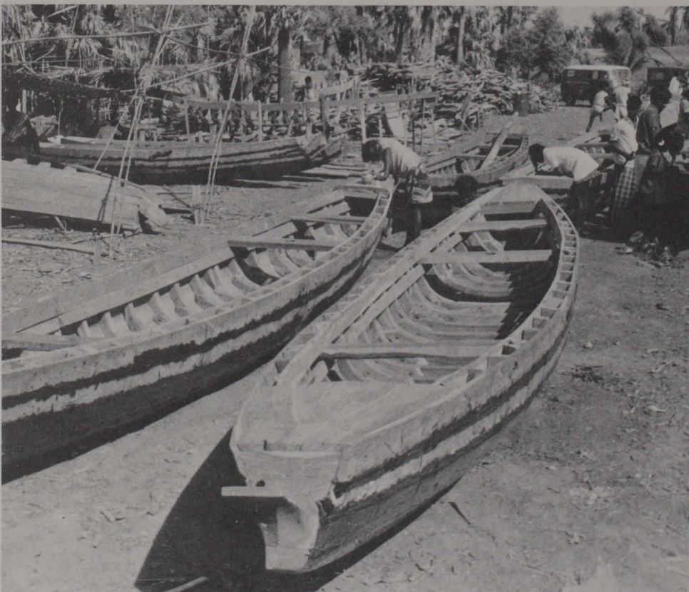
Members of the Gilakaladini Fishermen Cooperative Society constructing fishing boats to replace those lost in the recent cyclone which struck Andhra Pradesh. The project is financed by contributions from CARE OF CANADA, CIDA, and the State Government.
