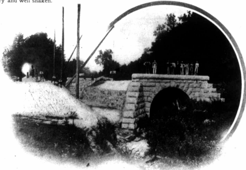
A Grand Trunk Railway Culvert, 20 foot opening, 205 feet long, near Port Hope, Ont. Wm. Gibson, Ex.-M.P., Contractor
