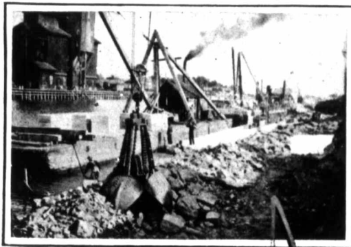
Ten Ton Concrete Blocks being placed in position on the Crib Work
